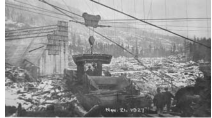
Construction of the South Slocan Dam, FortisBC Collection (West Kootenay Power & Light Co. Ltd.)
